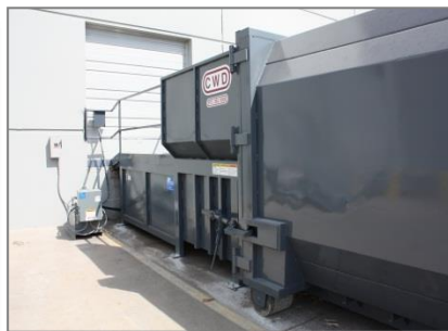
2-yard stationary compactor with a 40-cubic yard receiving container
