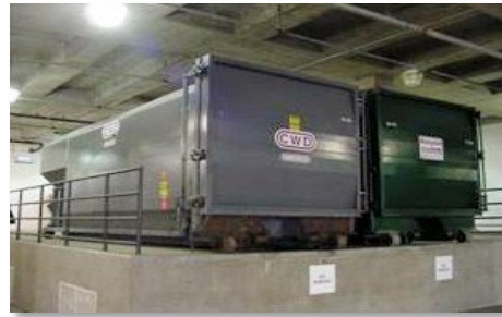
35 yard trash & recycle compactors in dock area
