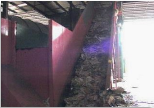
Conveyor moving newspaper to Trommel
