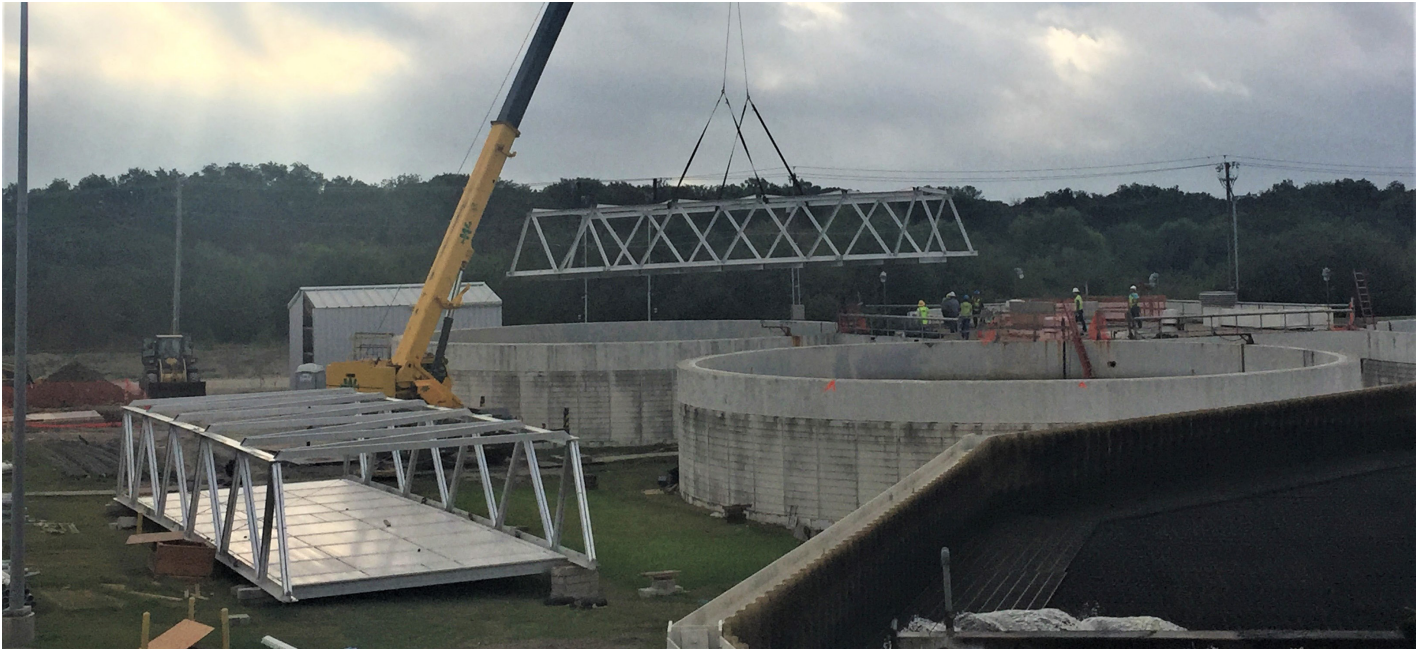
Rowlett Creek WWTP
